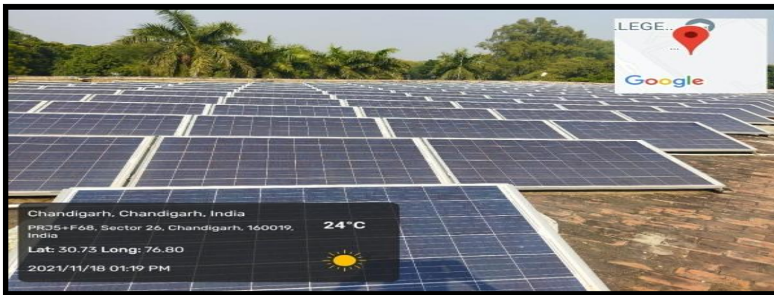
Solar Panels on the rooftop of Boys Hostel of the College
