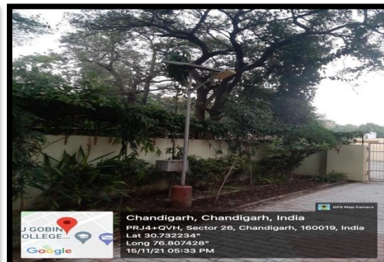
Solar Light in Boys Hostel
